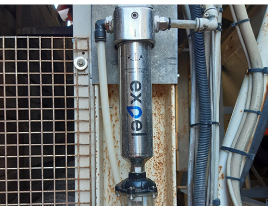
AVG EXPEL Compressed Air Filter installed
